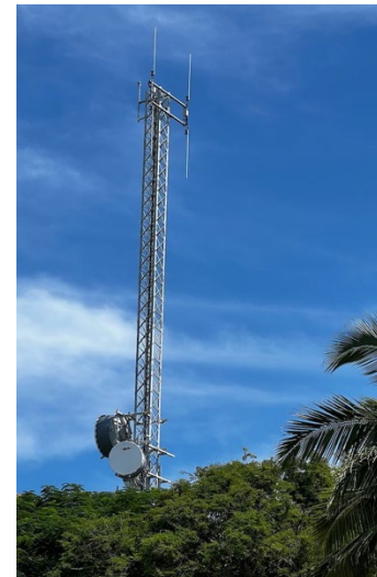
Figure 10: Telstra mobile tower in Medige Village
