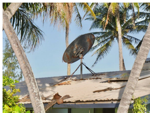
Figure 19: The proximity to salt water in Erub causes rapid corrosion of satellite dishes
