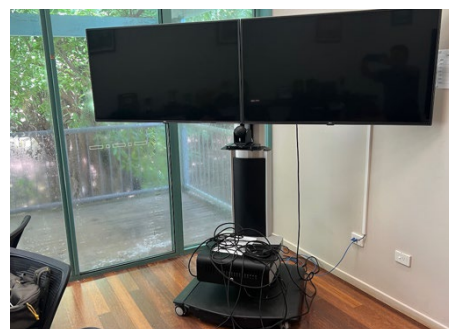
Figure 18: Videoconference facility in TSIRC Boardroom
