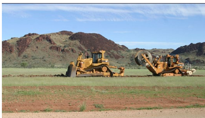
Figure 7: The fibre optic cable being laid near Blackstone community (Photo: Daniel Featherstone/ Ngaanyatjarra Media)
